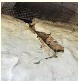
Crack on west wall.
