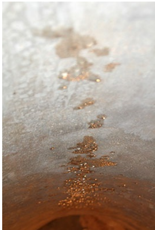
Moisture Damage in Crypt
