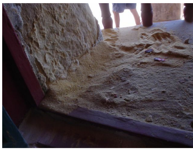
Pillar and door damage at Old Mission Santa Barbara. Photo Courtesy of SB Mission.
