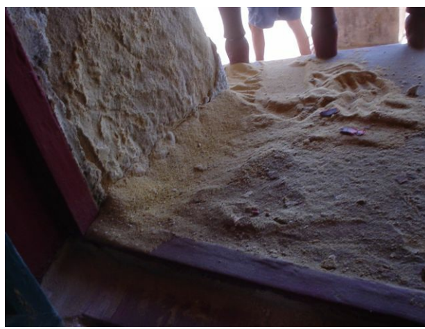
Pillar and door damage at Old Mission Santa Barbara. Photo Courtesy of SB Mission.
