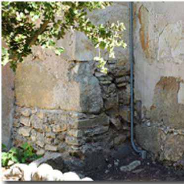
Detail view of crumbling wall
